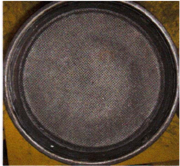
Inlet has an uneven gray appearance from thermal heat. The dark areas are minimal and acceptable.
